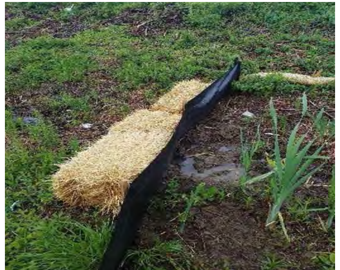
Fig 4: Straw bales near Str. F107-137 need to be staked in. Viewing south.
