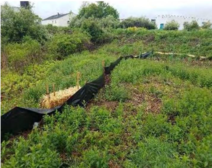
Fig 3: Silt fence near Str. F107-137, requires minimal repairs. Viewing south.
