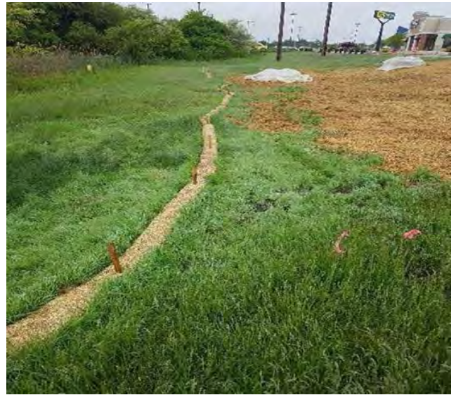
Fig 2: Straw waddle installed around Str. F107-135. Viewing southwest.
